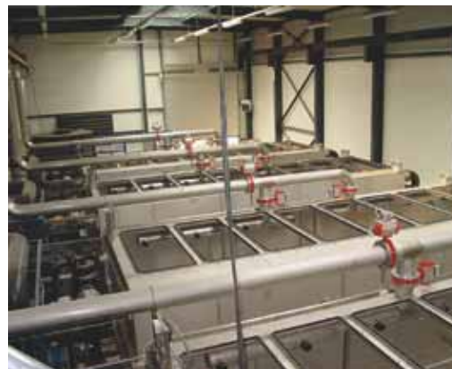
The Schilde WWTP, first MBR plant in Belgium, was commissioned in 2003 (courtesy of Aquafin).
